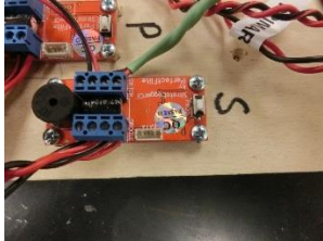
Altimeters(Primary and Secondary)
